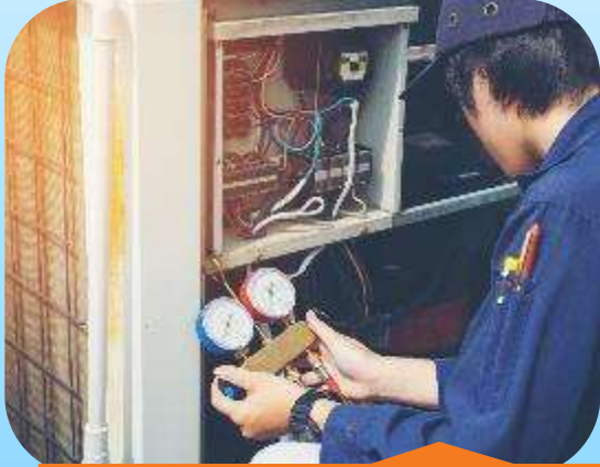
HVAC Quality Install
